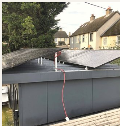
06 Garden rooms are suitable for solar panel installations to support an A rating
